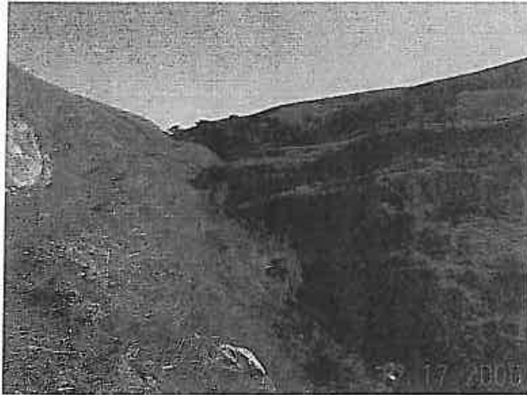
Photo 2-4. Active head-cut erosion advances upstream in this reach alongside the access road. As the stream down-cuts, stream banks, road embankment, and adjacent hillsides are weakened and made more erosion-prone. Use of placed rock, native willow plant material, and plantings of trees, shrubs, grasses, and grass-like plants should be used to check head-cuts, stabilize stream banks, and restore shade and habitat.
