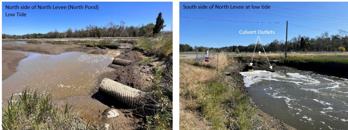
Figure 7. Existing Conditions: Culverts at the San Francisco Bay Trail at North Slough at Low Tide
