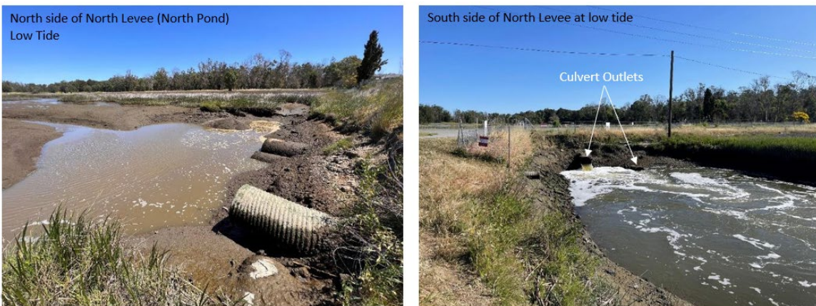
Figure 13 Existing Conditions: Culverts at the San Francisco Bay Trail at North Slough at Low Tide
