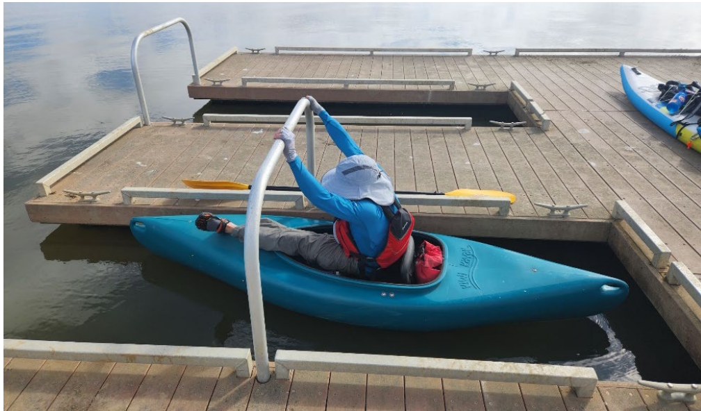
Figure 22 Example Finger dock with grab bar and toe boards at Cullinan Ranch Boat Launch, Napa County
